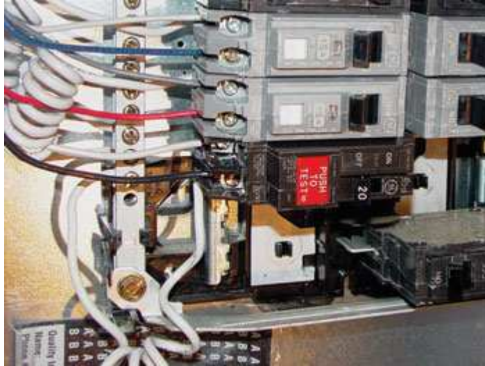
Photo 2. Typical GFCI overcurrent device
