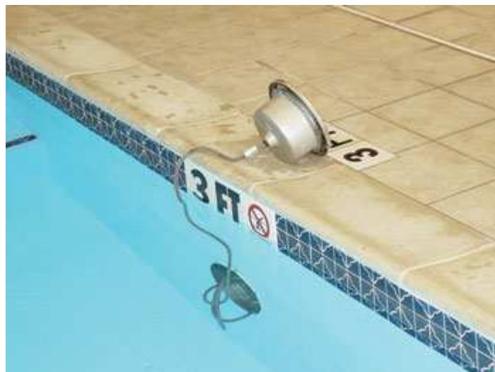
Photo 3. Underwater luminaires require GFCI protection.
